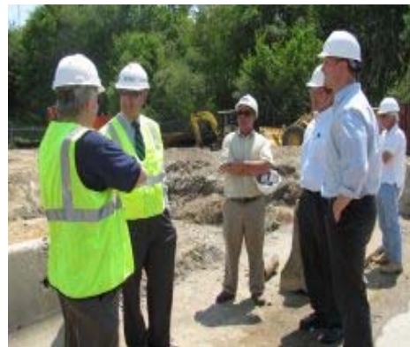
Example: Water Pollution Control Facility Upgrade in Fairhaven, MA
