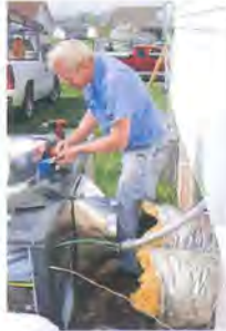
An efficient heat pump sized right for your home can be a real energy-saver!
